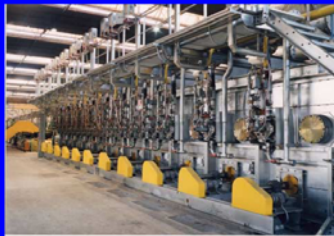
Steel, 30 t/h Tube Reheating
